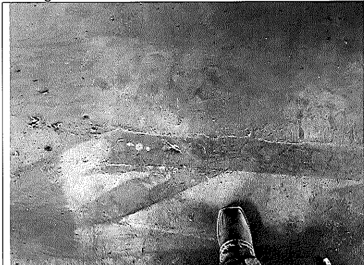
6. View of the ACM black mastic floor glue located throughout the east retail area and west first-floor level.
