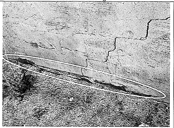
5. View of the ACM exterior wall patch on the north wall of Building C.
