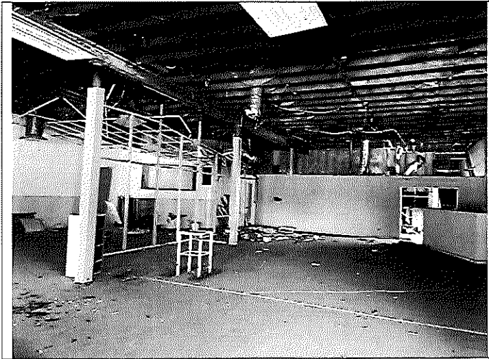
2. View of the inside of the east retail area inside Building A.
