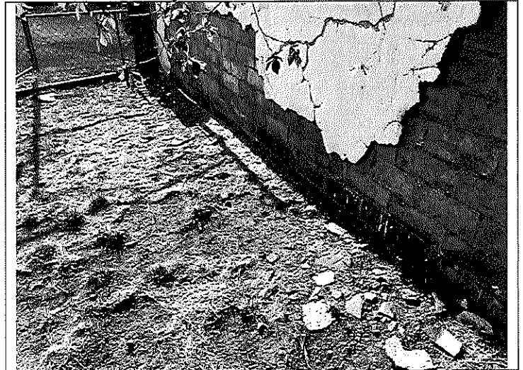
12. View of the ACM exterior wall plaster debris on the ground south of Building A.
