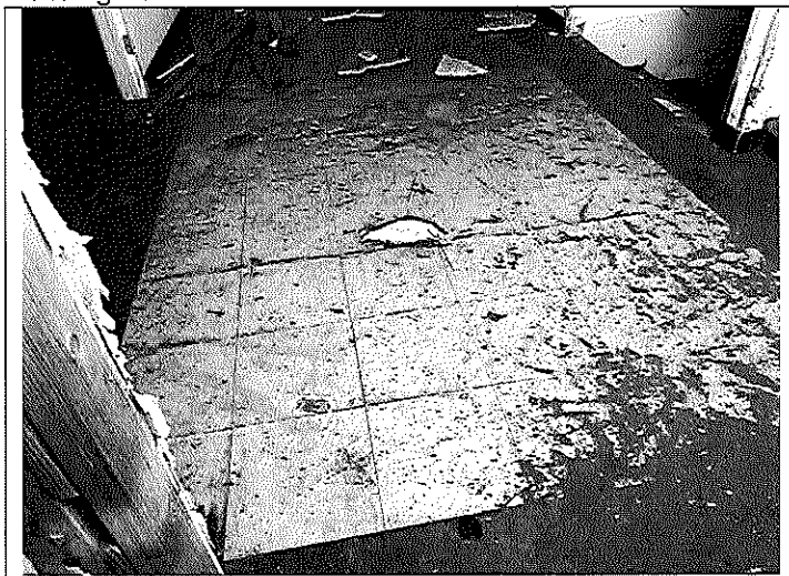
5. View of the 12"x12" Vinyl floor tile (black/white, mottled) associated with the ACM black mastic in the central hallway of Building A.
