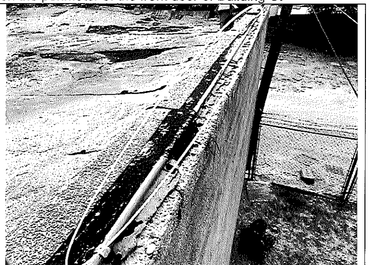
6. View of ACM parapet roof tar (black on the roof perimeter of Building C.
