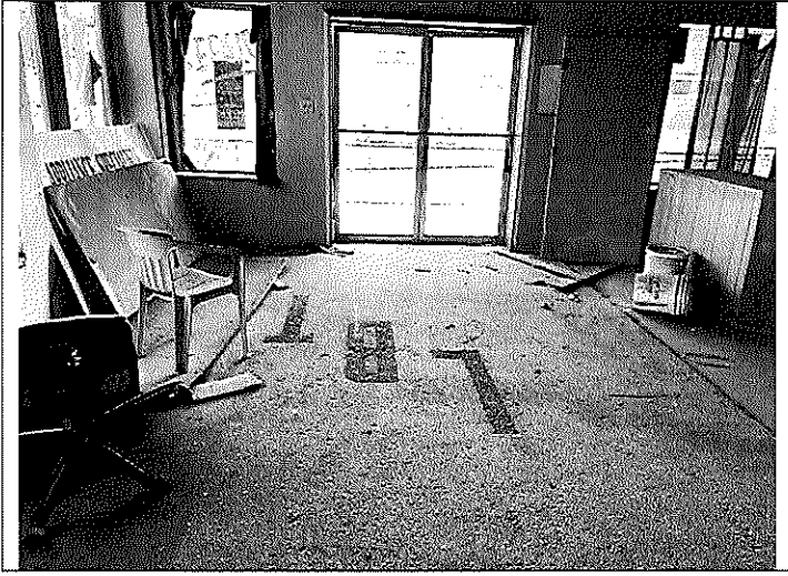
7. View of the poured flooring associated with the ACM black mastic in the NE foyer area of Building A.
