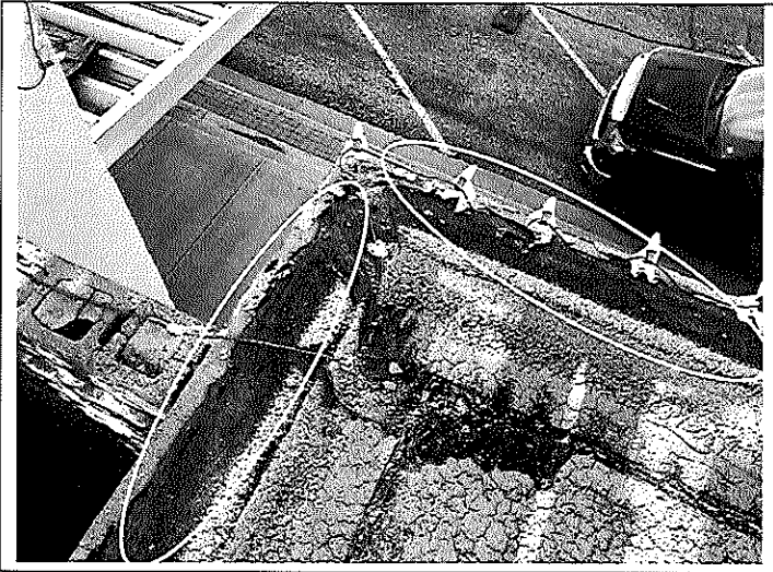
7. View of the ACM parapet roof tar on the roof of Building B.
