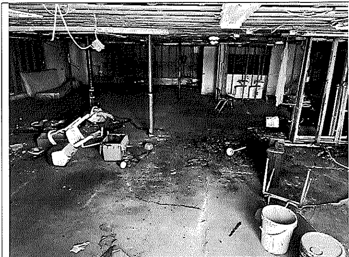
4. View of the first-floor level space in the west side of Building A.
