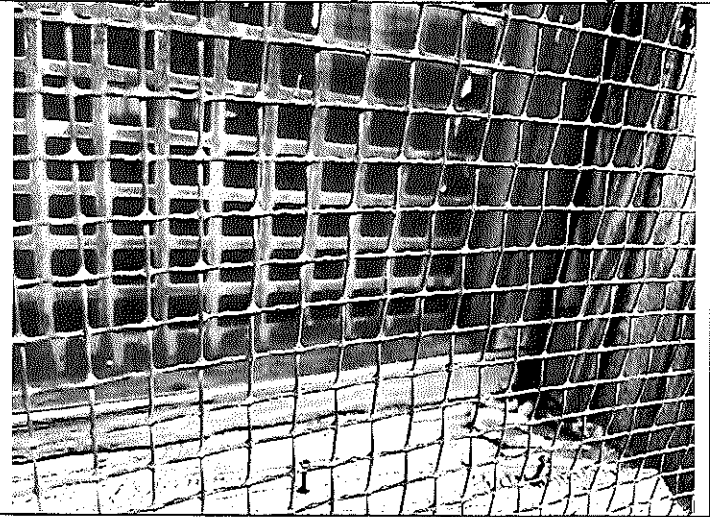
3. Close-up view of the ACM exterior door and window caulk on the west window of Building C
