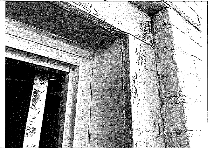
4. View of the ACM exterior door and window caulk (gray) on the perimeter of the front door of Building C.
