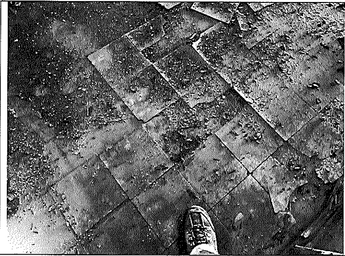
1. View of the ACM 9"x9" vinyl floor tile (beige, mottled) & black mastic on the floor along the north wall in Bldg. C.
