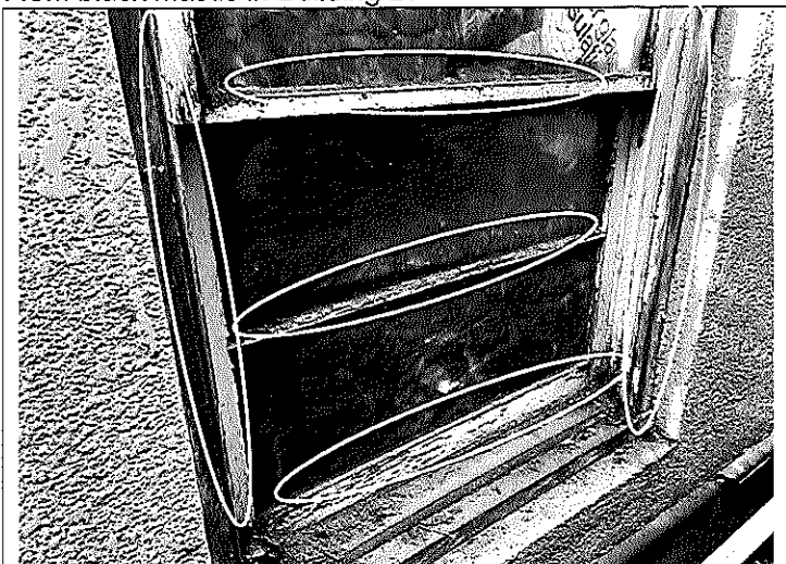
6. View of ACM window glazing and caulk on a typical historic perimeter window associated with Building B.
